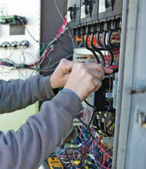
Maintenance worker Pete Biggs checks thermal overload circuits at the Houston Road Pump Station in Florence.
