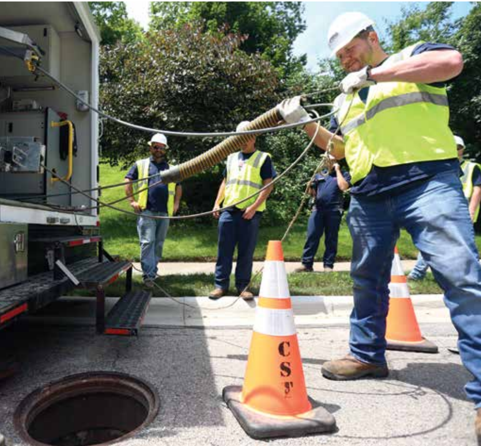
Bucky Skaggs (right) sets up for a sewer main inspection in Columbus, Ohio.
