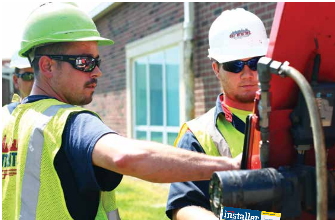
Dustin Robson (left) and Michael Snider make adjustments while jetting a drainline for Fairmoor Elementary School in Columbus, Ohio.
