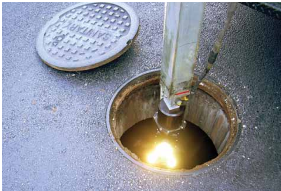
During the deployment of the CUES/IMX camera, each manhole and pipeline will be inspected and recorded on electronic media.
