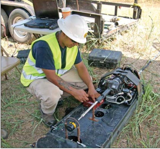
A technician in the field readies the FlyEye system for an inspection of an interceptor.
