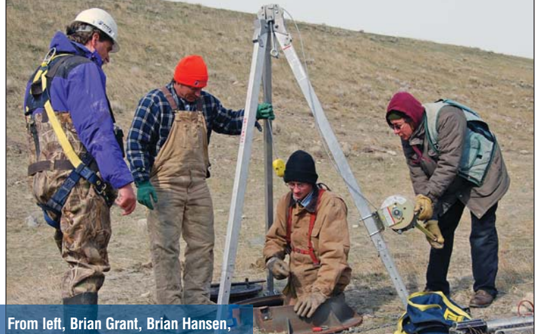
From left, Brian Grant, Brian Hansen, Eldon Lambert and Randy Laskowski make final preparations before placing a camera for inspection in a manhole at Martinsdale Dam in Montana.
