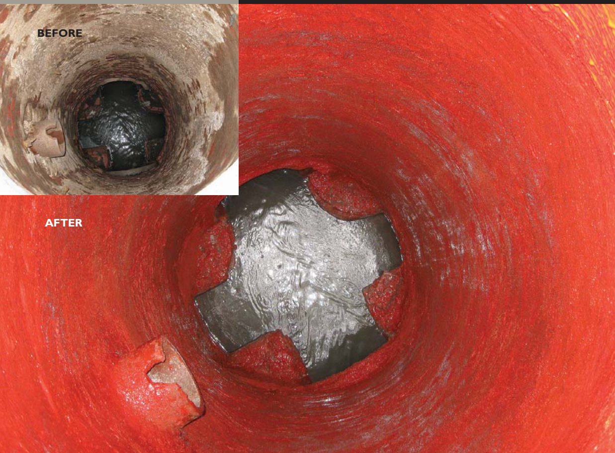
A manhole is shown before and after lining with the epoxy coating system. (Photos courtesy Wastewater Collection Division, Miami-Dade Water and Sewer Department)
