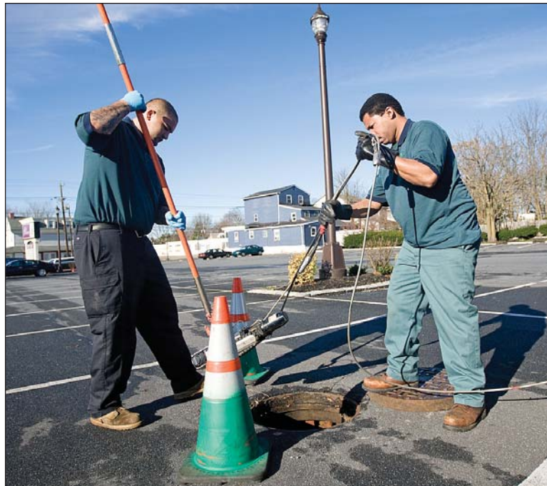
Drain Visions technicians J.R. Moore and Mike Beausil retrieve an inspection camera after a job in Blackwood, N.J.
