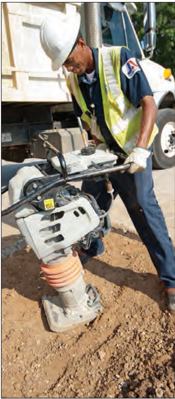
Utility technician Aaron Hillard tamps the soil with a Multiquip tamper after connecting a new service line.
